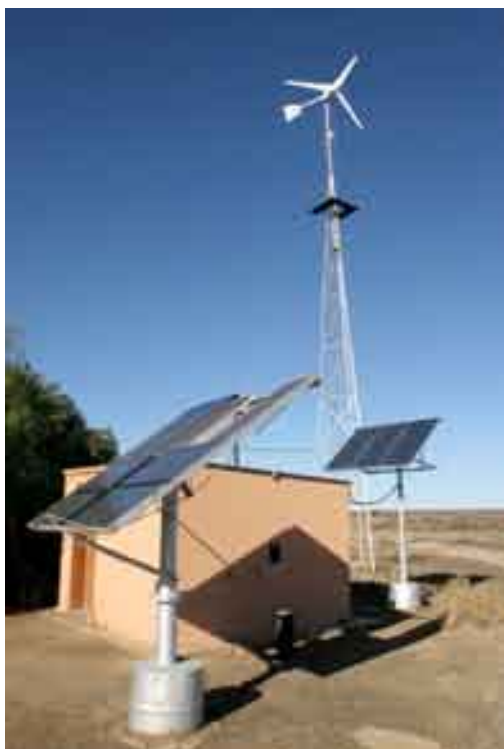
Solar panels and a wind turbine on a farm near Verneukpan in the arid Northern Cape. Johann van Tonder/PictureNET Africa
