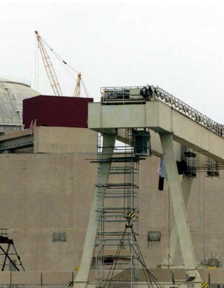
Iran's nuclear power plant at Boushehr ... before the revolution, the US was closely involved in Iran's nuclear programme. AP Photo/Vahid Salemi
